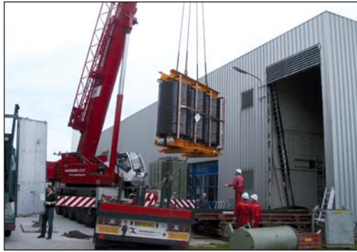
Figure 3: Hoisting of the new transformer into the machinery hall of the LLF
